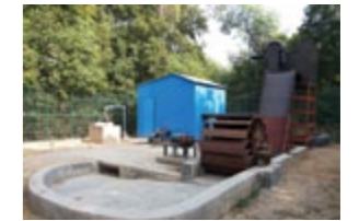
Fig. 9 Overall view of Ultra-micro hydel power package
