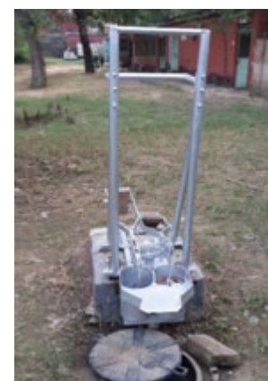
Fig. 18 Improved treadle pump installed at Micromodel lab.
